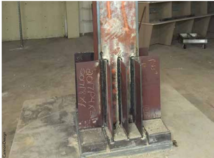
New base plates transfer column loads to enlarged footings at the basement level.
