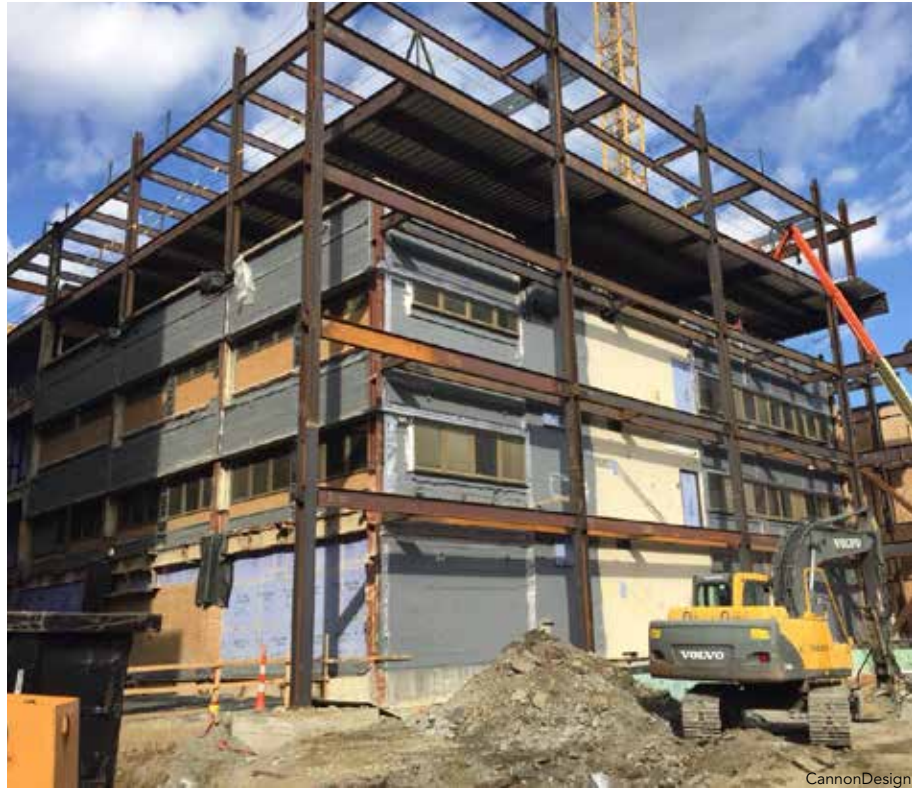
The original Stauffer wing remained operational as it was encapsulated by the new steel framing.
