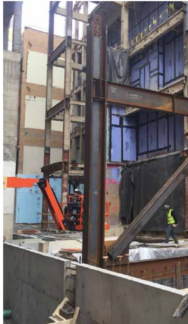
Braced frames and moment frames serve as the new lateral force-resisting system.
