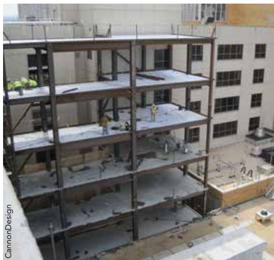
A nine-story steel-framed link building connects the new addition to the existing hospital campus.
