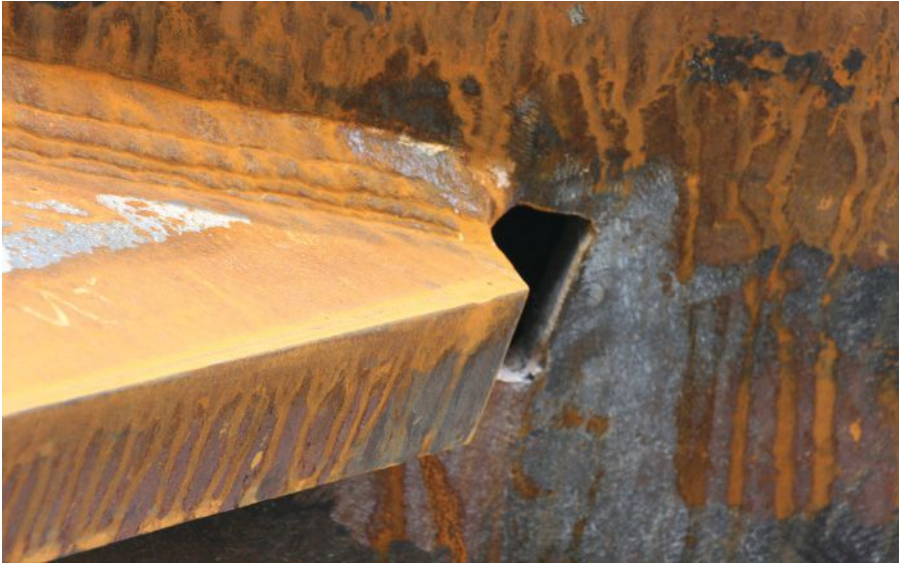
left: A rectangular slot cut into an HSS seismic brace wall, for fitting onto a gusset plate.
