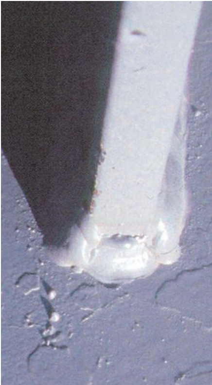
An example of notches and poor quality welding around the end of stiffeners and connection plates.
