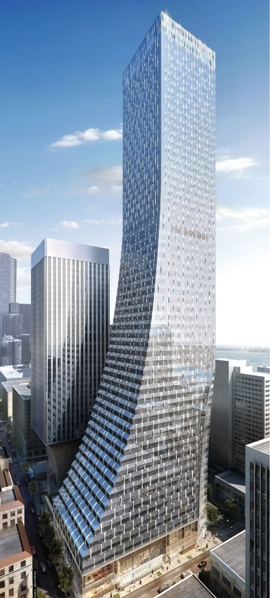
The ongoing Rainier Square project in Seattle, which is being built using the SpeedCore system.
