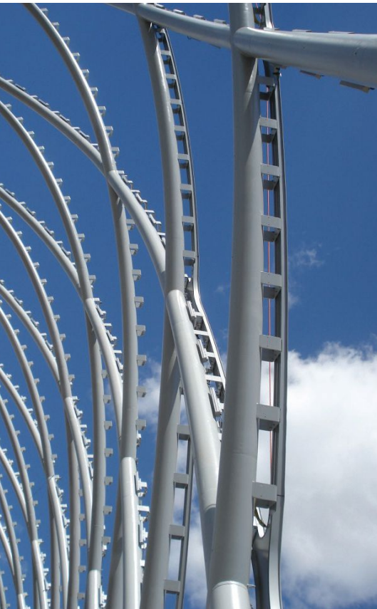
The roof of the Anaheim Regional Transportation Intermodal Center employs 14-in.-diameter curved, interlocking HSS to form a diagrid shell.
