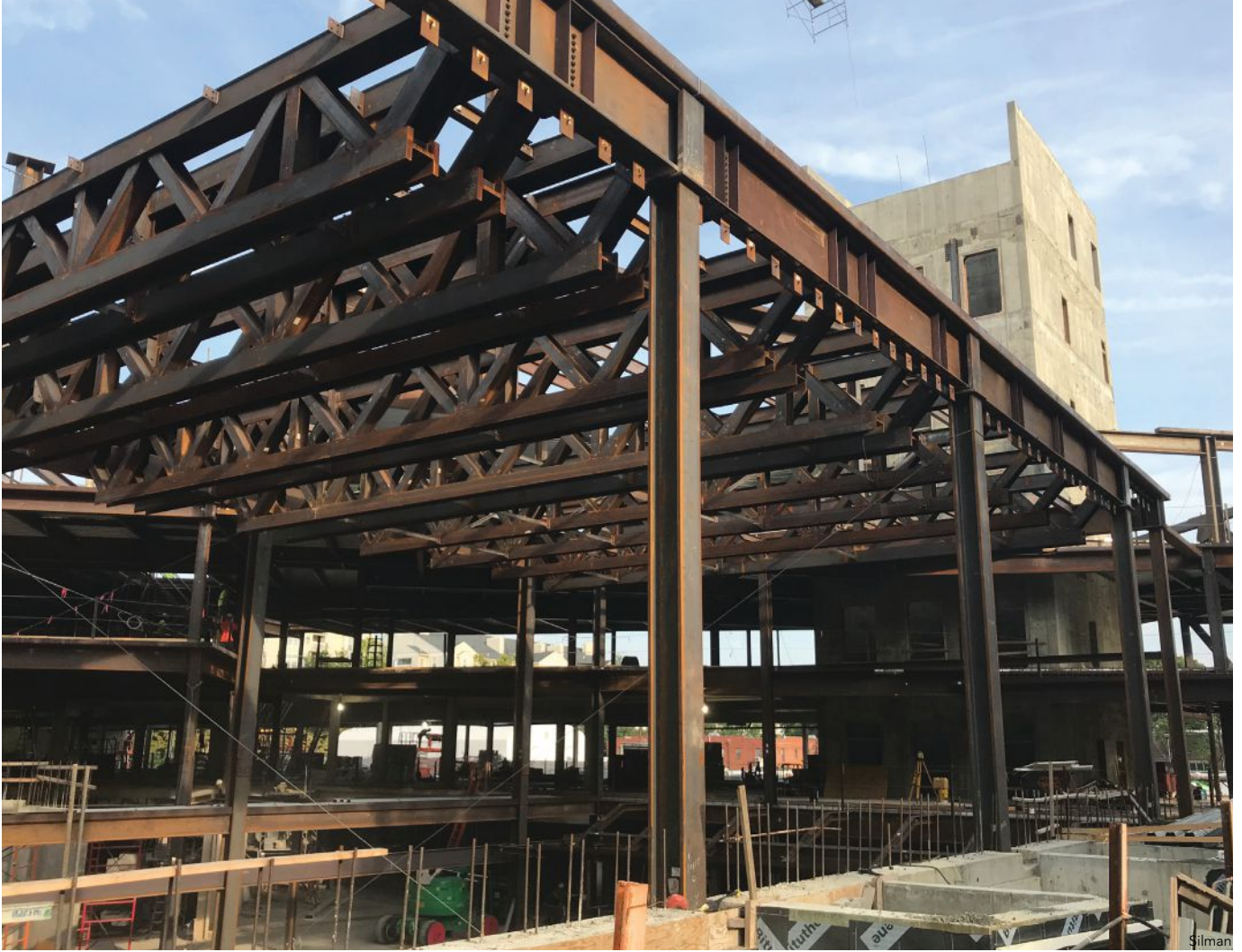
Above the theater, trusses were the optimal solution to meet the needs of future expansion, MEP routing, and allowable floor depths.
