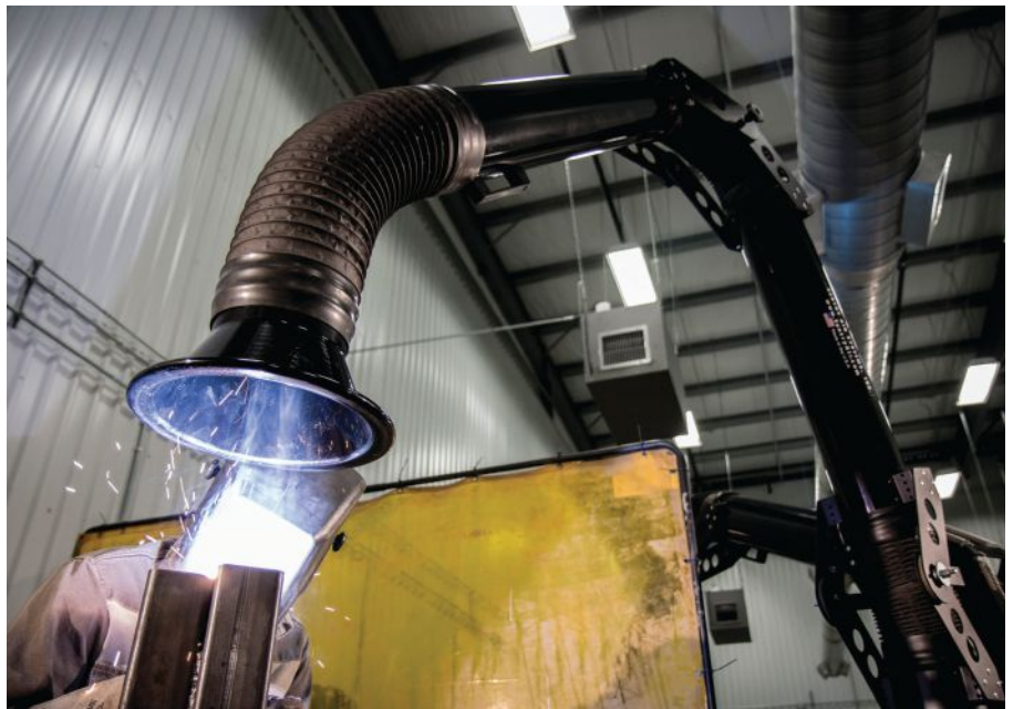
above: A worker welds next to a dual-operator, portable welding fume extractor featuring heavy-duty arms and a cleanable filter.
