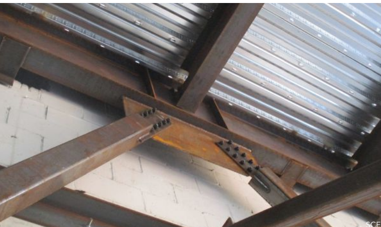
below: The engineering team introduced a new lateral load-resisting system consisting of chevron braces, with one chevron brace being added to each face of the main studio area.
