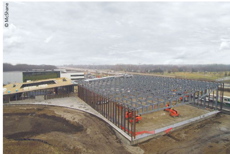
below: The facility consists of two attached buildings topped by a gently sloping continuous mono-pitch roof.
