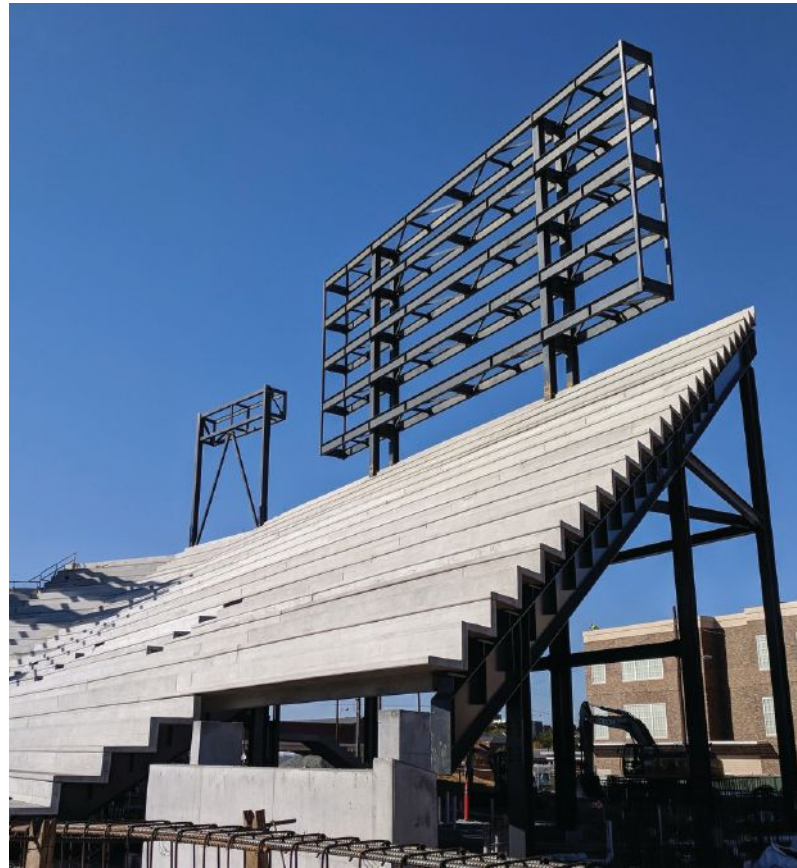
below: The scoreboard, located at the end of a raker cantilever, was fit up flat at grade and then erected with a single lift into its final position.
