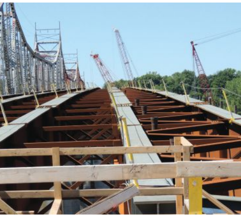
above: The secondary structural steel contained 346 cross frames, 336 lateral bracings, and 24 diaphragms.
