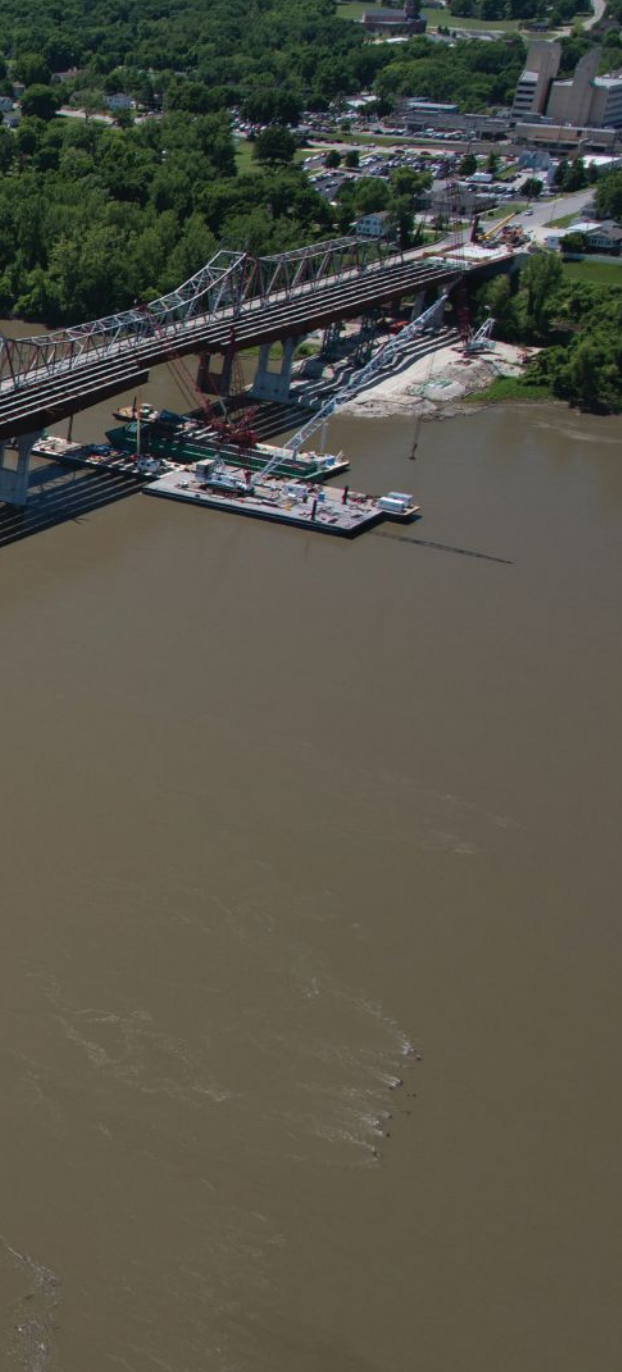
left: The superstructure for the new bridge, which uses 5,800 tons of structural steel in all, nearing completion.
