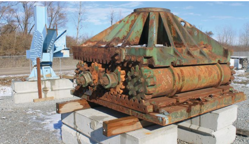
above: One of the more unique specimens at S-BRITE is this large nested roller bearing from one of the main river piers of the I-35W bridge.
