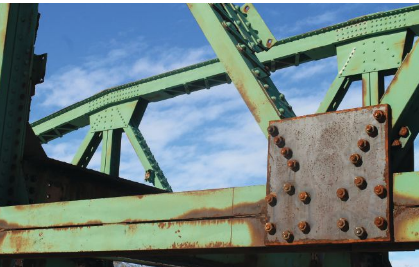
below: A close-up of the bolted splice used when S-BRITE engineers re-erected the Indian Trail Bridge.
