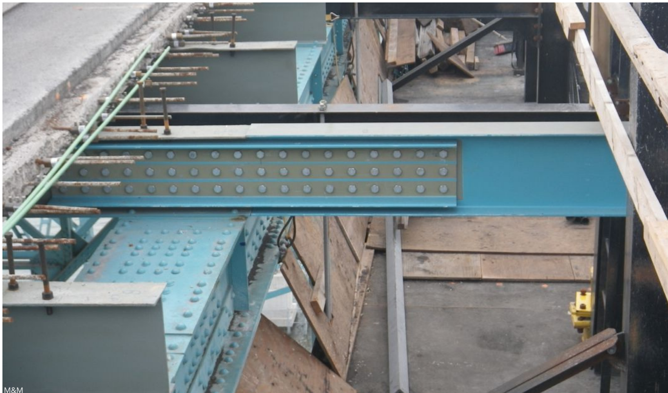
M&M A primer with a cure time of 19 hours was used on a steel railing replacement project on the Ambassador Bridge between Detroit and Windsor, Canada.
