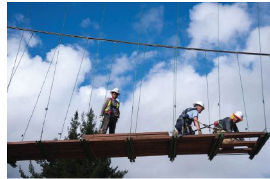
below: Craig Smart, John Hastings, and a B2P representative working the decking toward the middle of the bridge.
