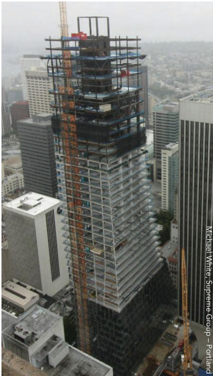
Rainier Square Tower in downtown Seattle, the first building to use the SpeedCore system.
