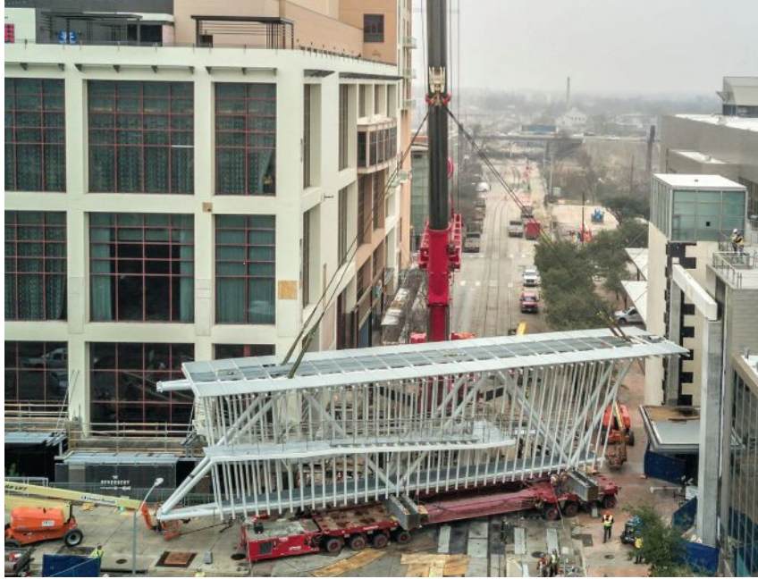
above and left: In the course of one weekend, the bridge was transported down 4th Street on self-propelled mobile transporters, where a 900-ton erection crane lifted it into place.
