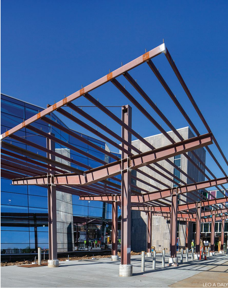
above: The main canopy structural system, 40 ft wide by 100 ft long, consists of wide-flange columns and built-up tapered WT members that vary from 24 in. in depth at center to 12 in. deep at the ends.
