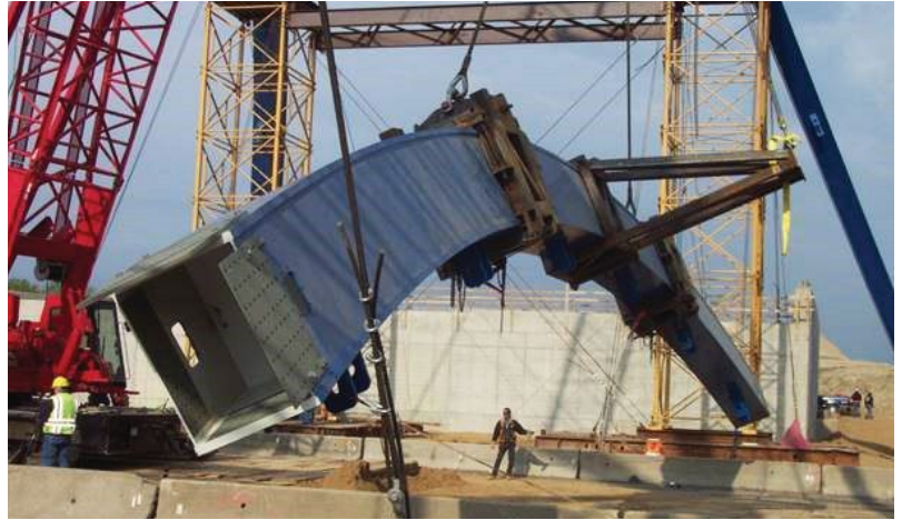
Clamping fixtures on the Interstate 94 Gateway Bridge arch section lift, a tied-arch bridge in Taylor, Mich.
