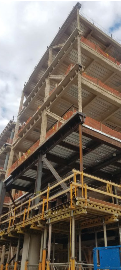
A view from the southwest, showing one of the building's vertically oriented trusses.
