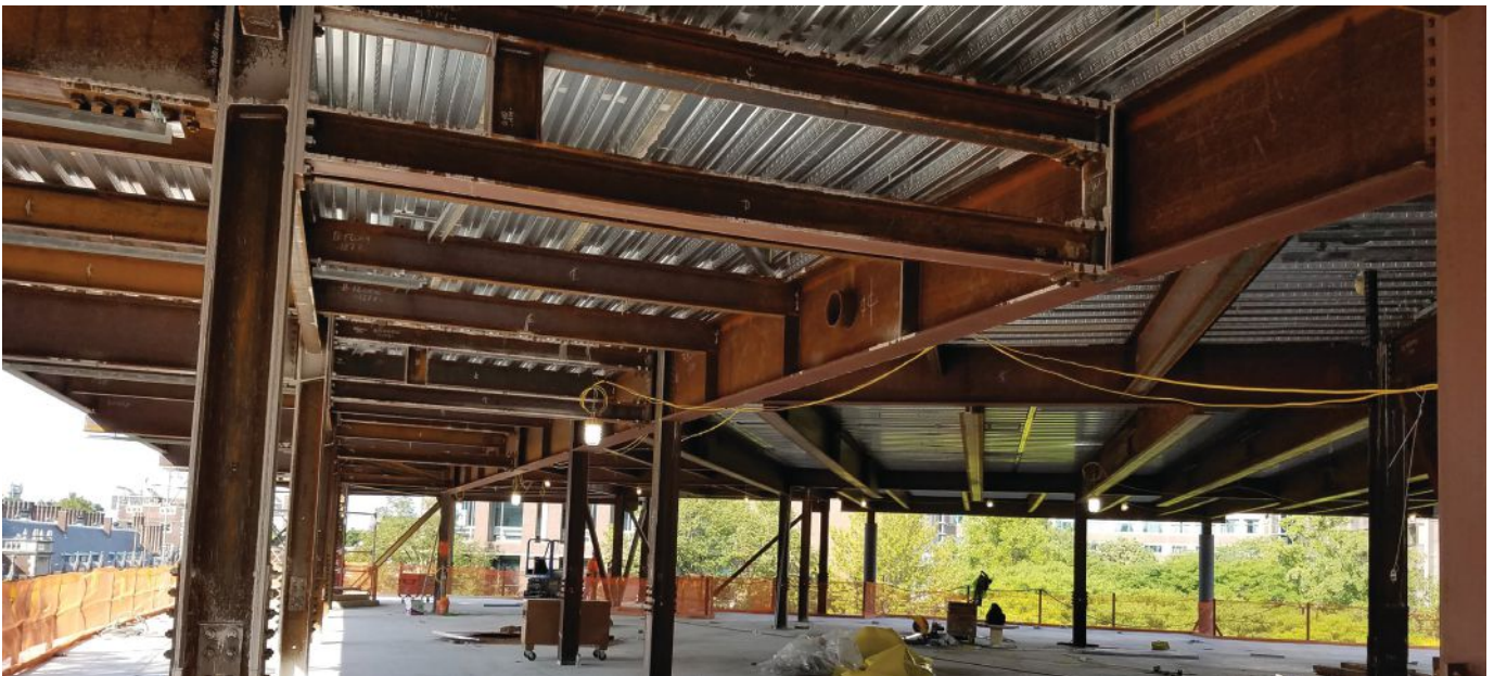
opposite page and below: The five-story building uses 467 tons of structural steel for its framing system.
