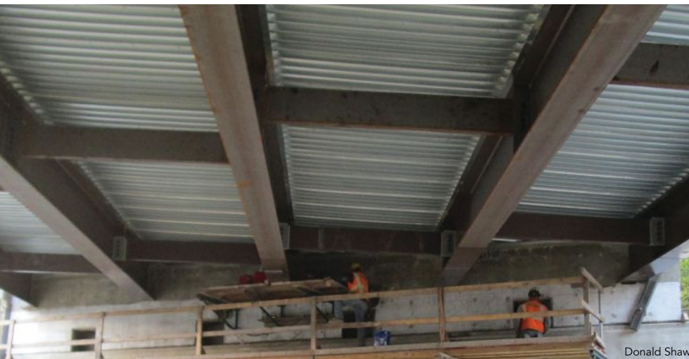
The steel bridge superstructure, made from W33x201 and concrete deck, includes five skewed 71-ft-long girders spaced at 9 ft, 9 in. apart, with four steel bracing elements per gap (16 in all).
