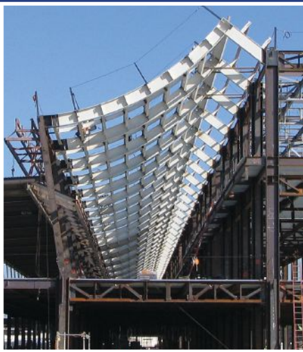
2011 IDEAS 2 National Winner - 420 tons of rectangular tubing, pipe and beams for the roof at the Norman Y. Mineta San Jose International Airport. San Jose, CA
