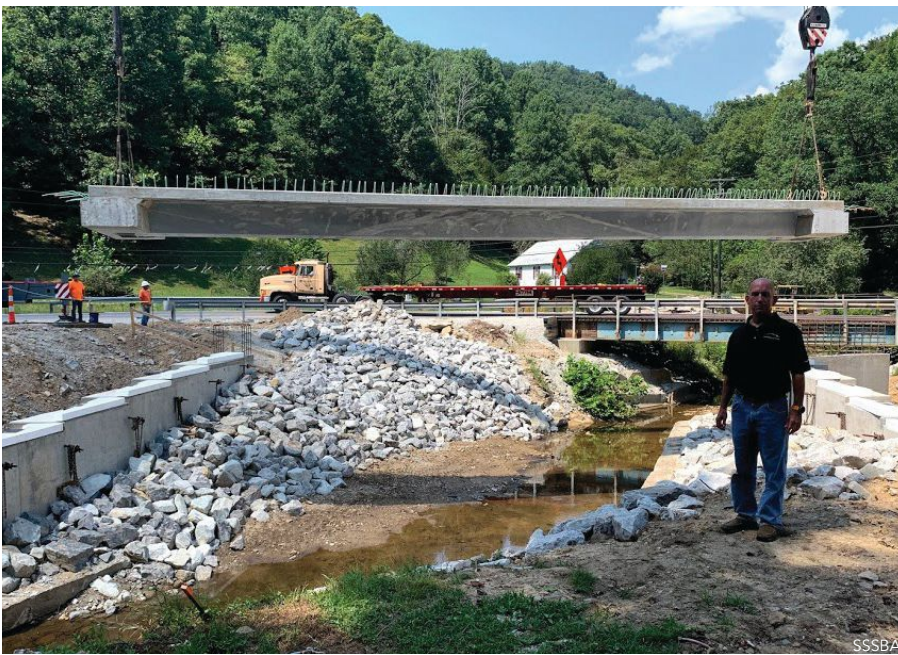
opposite page and above: Installing the Fourteen Mile Bridge in Lincoln County (District 2) near East Lynn, W.V., a PBTG bridge. Comprehensive research, development, and proof-of-concept efforts for the PBTG design were led by West Virginia University and Marshall University.
