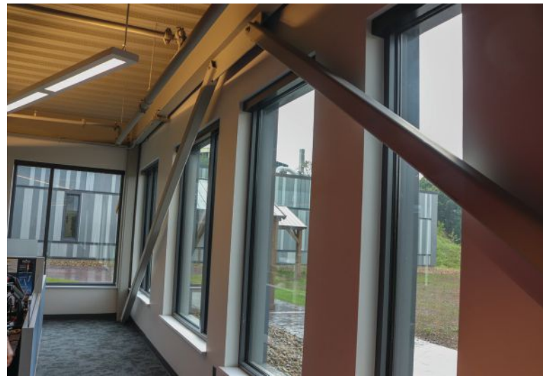
below: Exposed steel, such as the bracing below, was a primary design focus for the design team.
