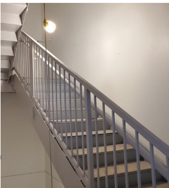
below: Another recent McGregor project, a stair for MIT's Kendall Square Initiative.
