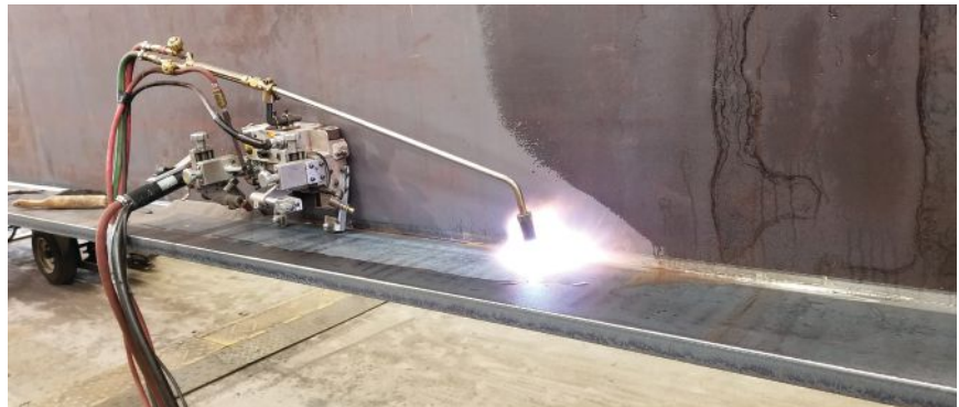
Fig. 6. Traditional box web-to-flange CJPs require backing, bevels, and multiple passes (above), while I-girder web-to-flange welds do not require bevels and backing and are usually done in one pass (below).
