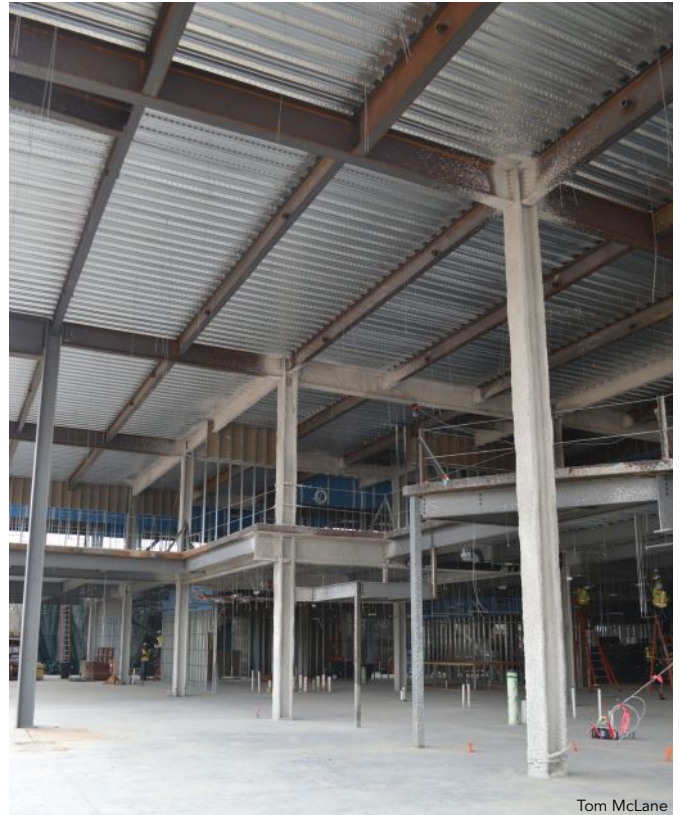
below: Framing for the main lobby during construction. The open, two-story lobby space features exposed steel columns with an AESS 1 (basic elements) finish.
