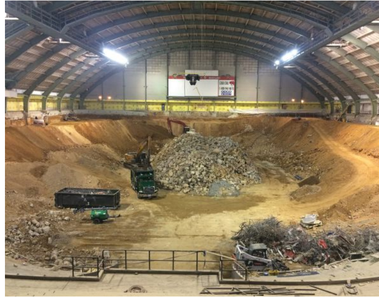
below: The arena seating bowl was demolished and excavated to accommodate the new football practice field.
