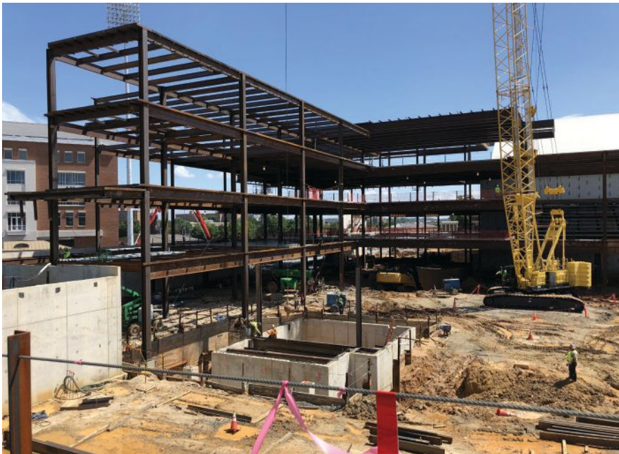
left: More than 2,261 tons of structural steel were used to construct the Center for Sports Medicine and Human Performance.
