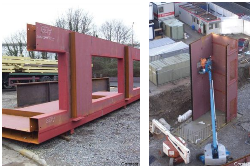
Fig. 6. A Corefast panel arriving at a site as a prefabricated unit (left) and being erected into a final configuration (right).
