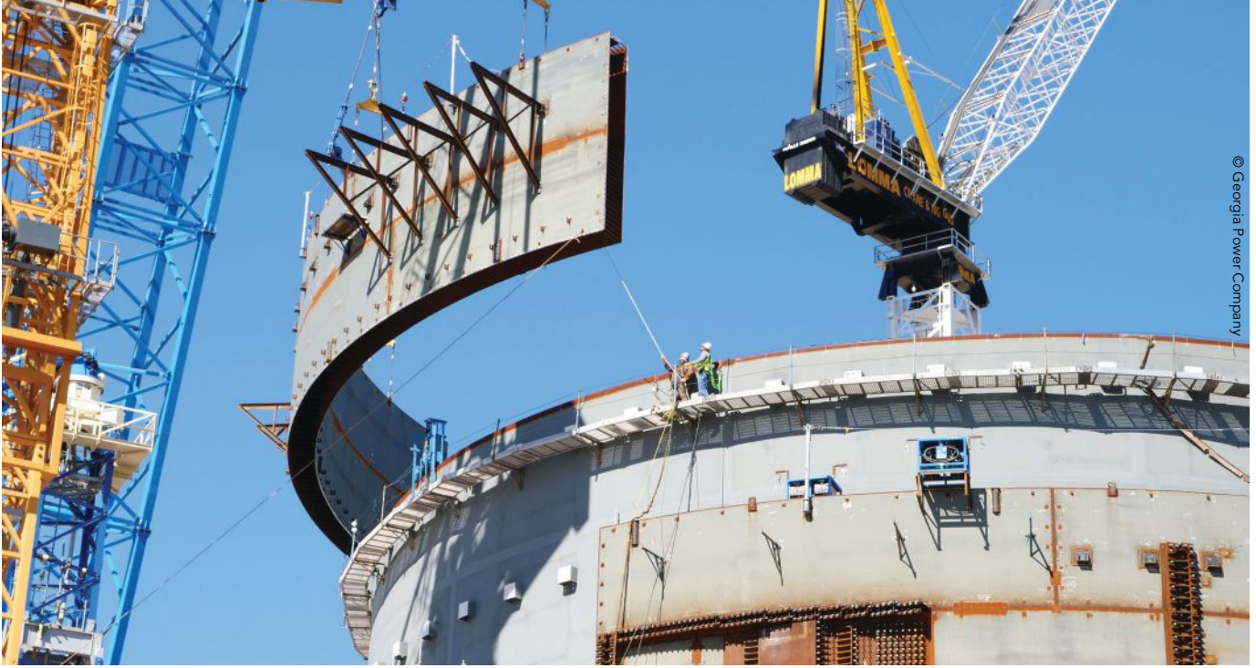
Fig. 7. Composite plate shear walls being used in the Vogtle Unit 3 Shield Building (a nuclear facility application).
