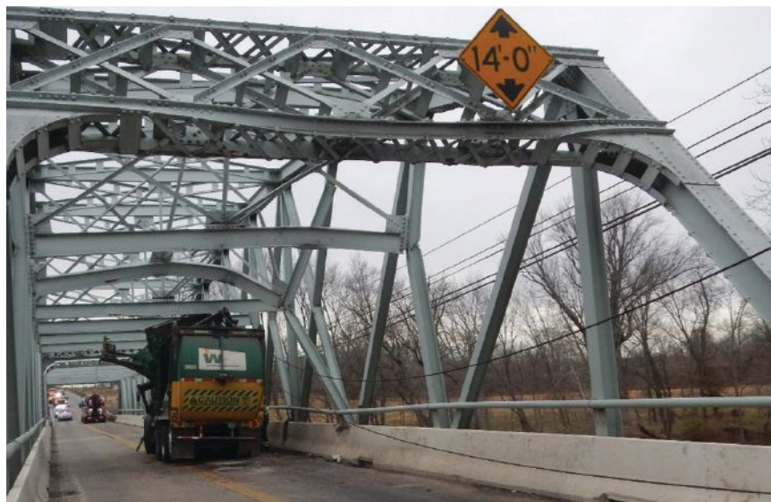
Fig. 3. Impact damage to through-truss struts by an over-height vehicle.
