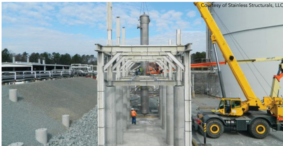
above: Structural stainless steels have been widely used in industrial process applications for many years. In this example, the framing system was fabricated from laser-fused stainless steel plate and will have an extremely long life span, even in a rugged, industrial environment.
