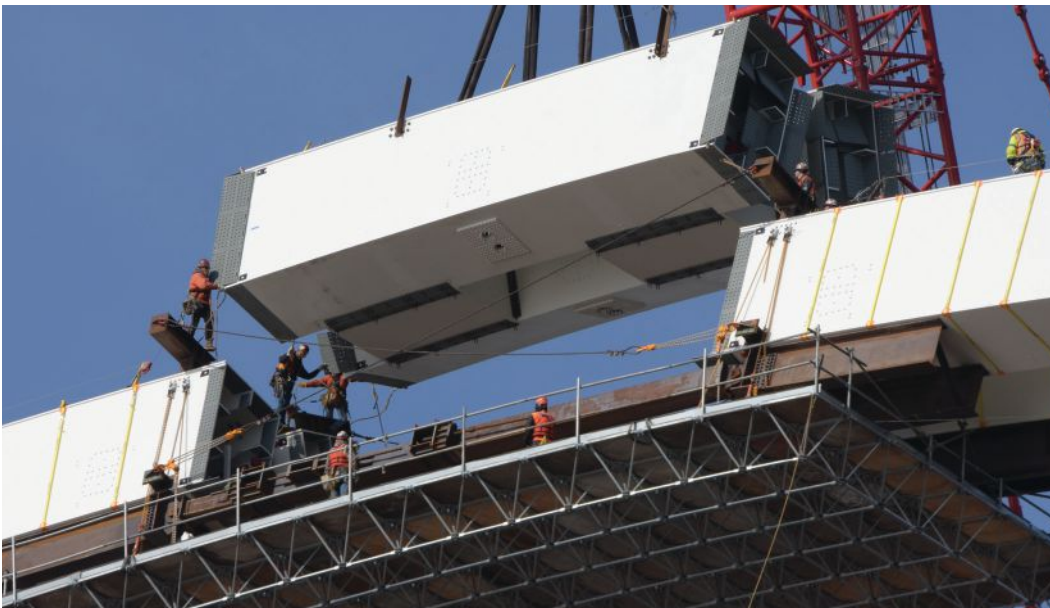
above: Installing struts to help with keystone installation for the westbound arch.
