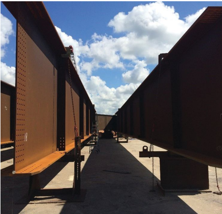
below: Complete shop assembly was key to avoiding fit-up issues and delays at the project site.
