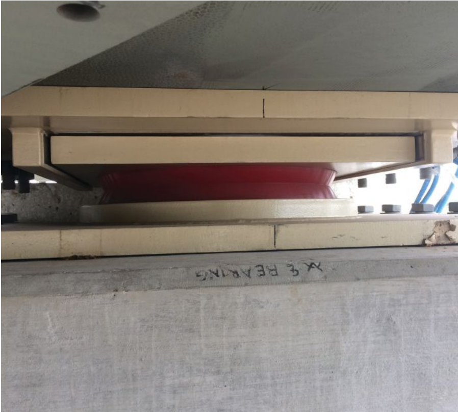
above: The straddle bent is supported by three custom-fabricated 5-ft, 2-in.-diameter disc bearings with a maximum supported service load of over 3,500 tons.
