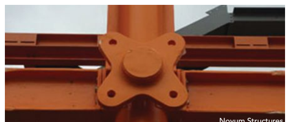
A connection at a hospital project.
