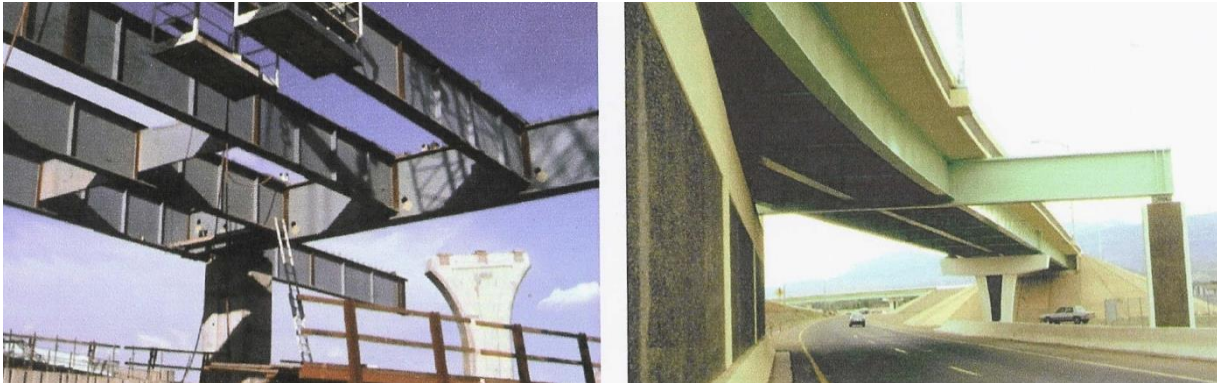
Figure 16. Straddle bents with integral steel pier caps (Abu-Hawash et al. 2005) (courtesy of Iowa DOT, HDR Engineering, and NSBA).
