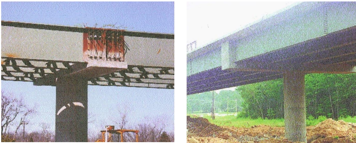
Figure 15. Typical post-tensioned concrete integral bent cap with a single column pier (Wasserman 1997) (courtesy of Tennessee DOT and NSBA).
