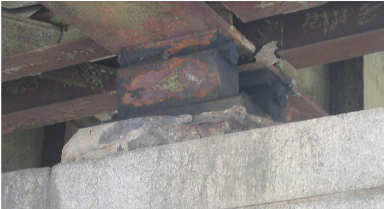
Figure 30. Photo. Corroded bearing.
