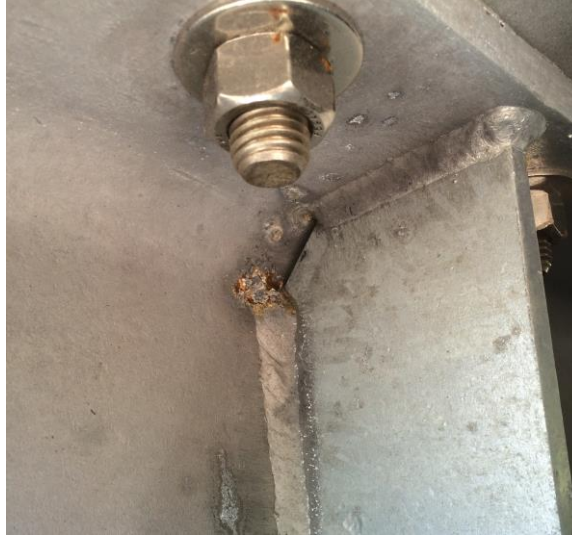
Figure 40. Photo. Connection plate welded to rolled I-beam along with corrosion emanating from unsealed weld.
