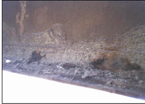
Figure 28. Photo. Heavy corrosion of bottom flange and web due to collection of poulitice.
