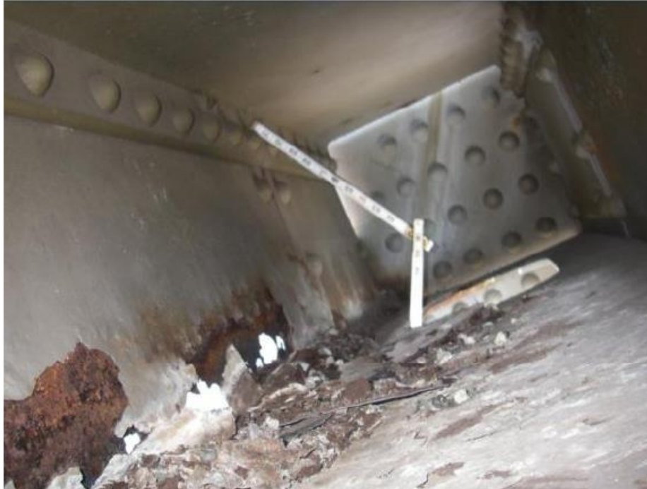
Figure 33. Photo. Inside of built-up box member.
