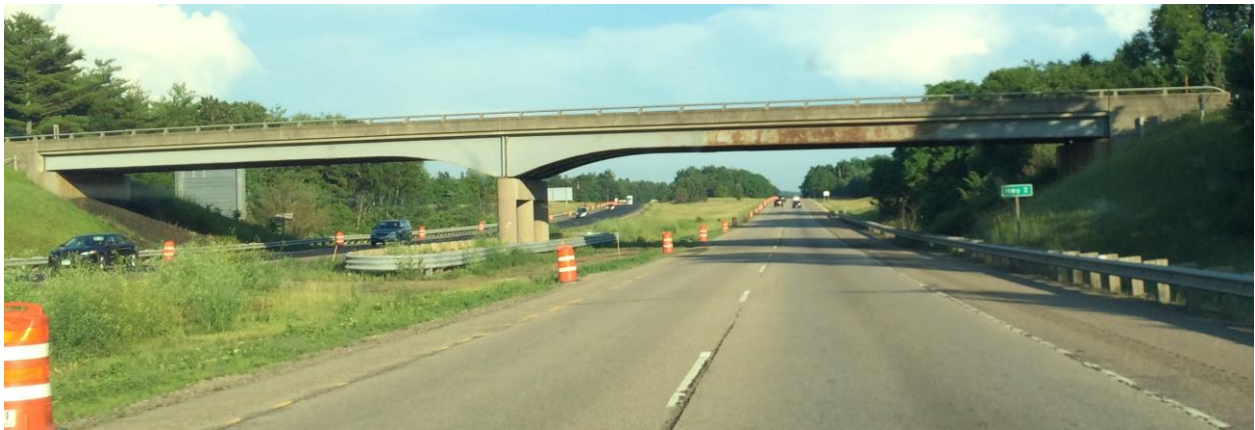
Figure 26. Photo. Accelerated corrosion on the inbound fascia girder of a grade separate structure, particularly over the right travel lane.
