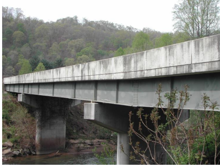
Figure 14. Photo. Bridge in West Virginia with a single-coat inorganic zinc-rich paint system after 25 years.
