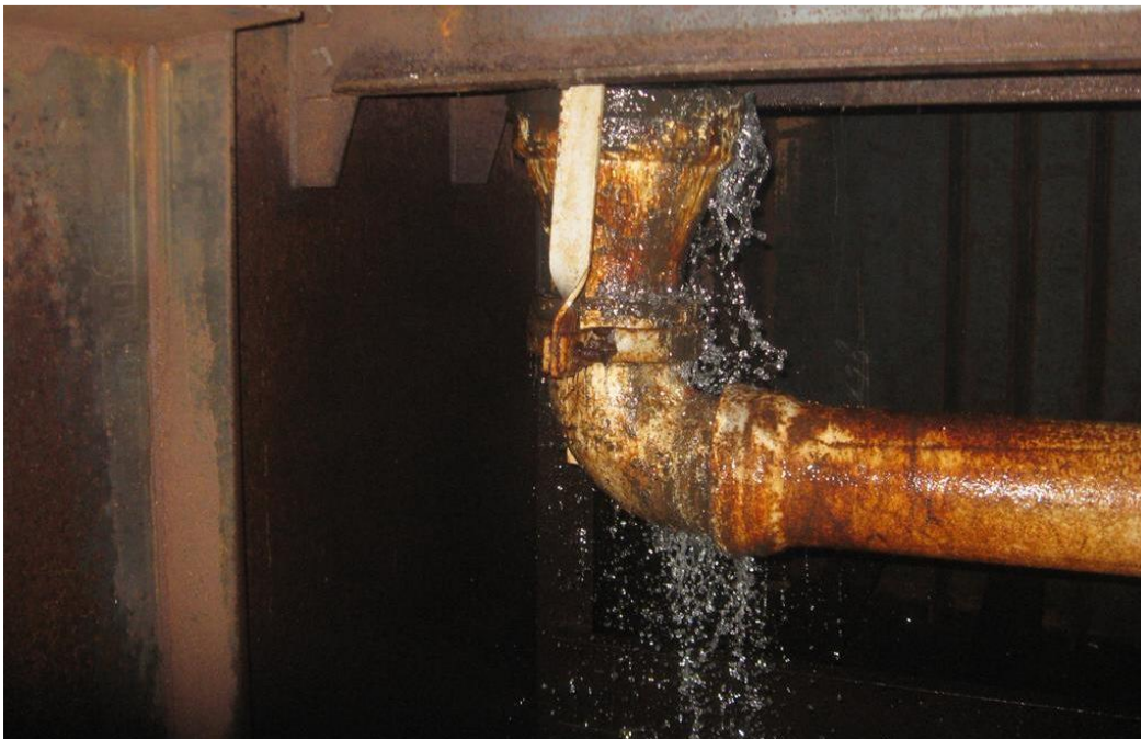
Figure 22. Photo. Clogged drain leaking water onto superstructure.
