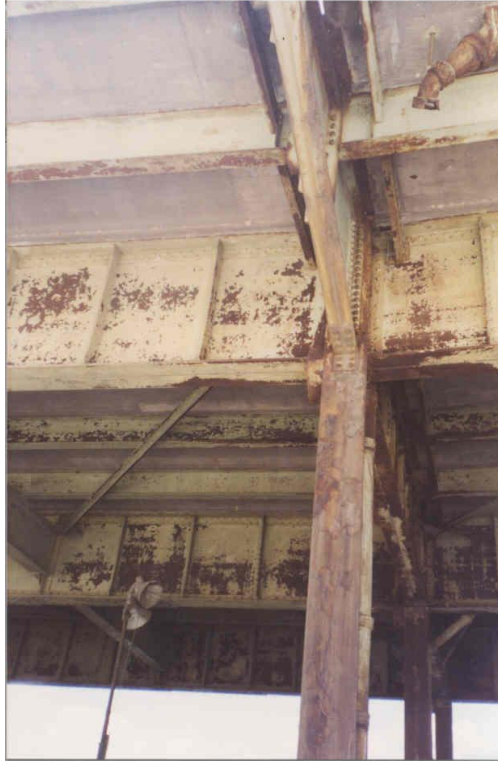
Figure 21. Photo. Missing portion of deck drain downspout.
