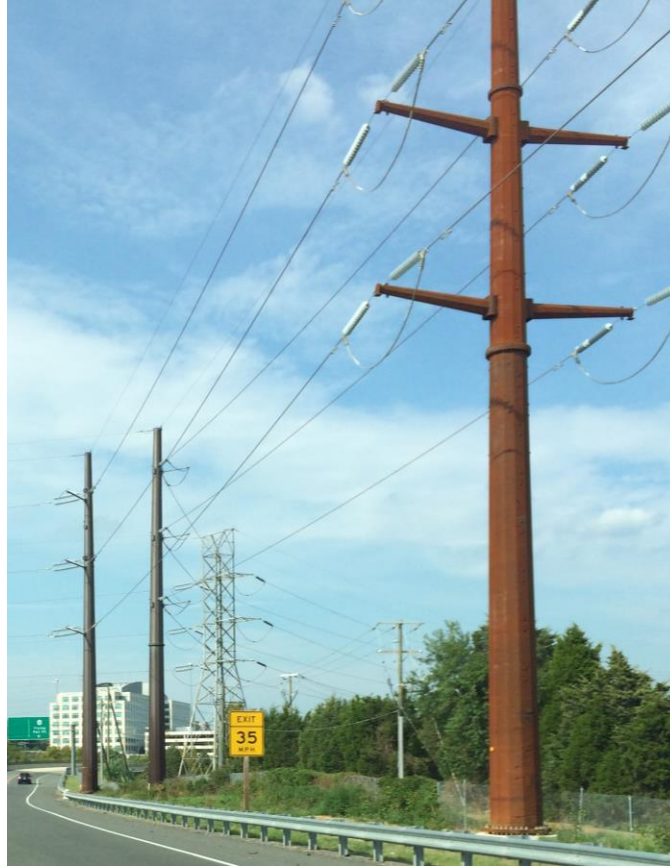
Figure 8. Photo. Different color of rust patina in new transmission tower (close) and older (far).
