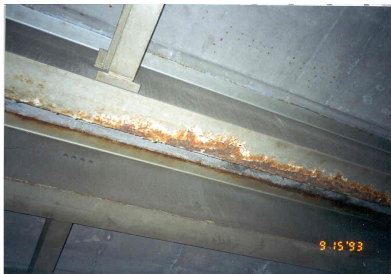
Figure 17. Photo. Steel directly beneath longitudinal expansion joints that have leaked corrosive runoff from the deck.
