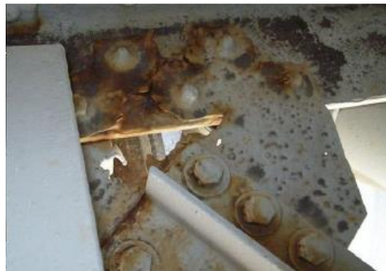
Figure 38. Photo. Corroded lateral gusset plate detail.
