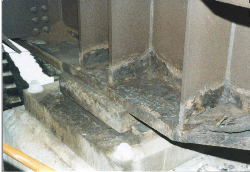
Figure 34. Photo. Girder end on a bearing below a leaking deck joint. Horizontal flange and vertical stiffeners create an excellent trap for debris and moisture.
