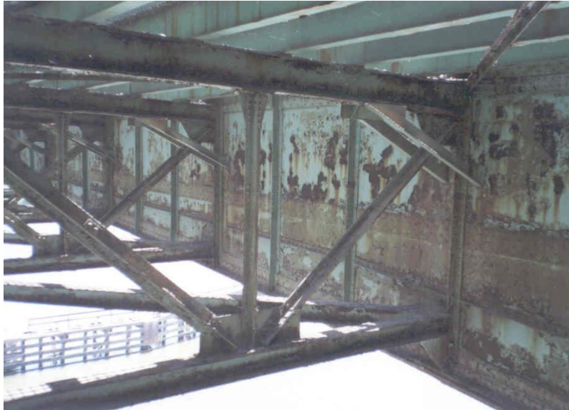
Figure 20. Photo. The area under an open grid deck acting as one large leaking joint.
