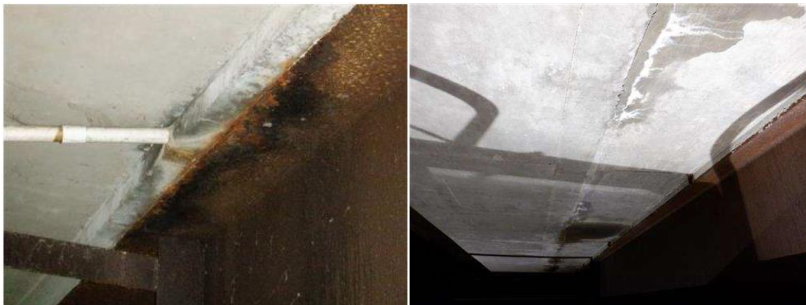
Figure 13. Examples of In-Span Leaking Noted in Bridges
