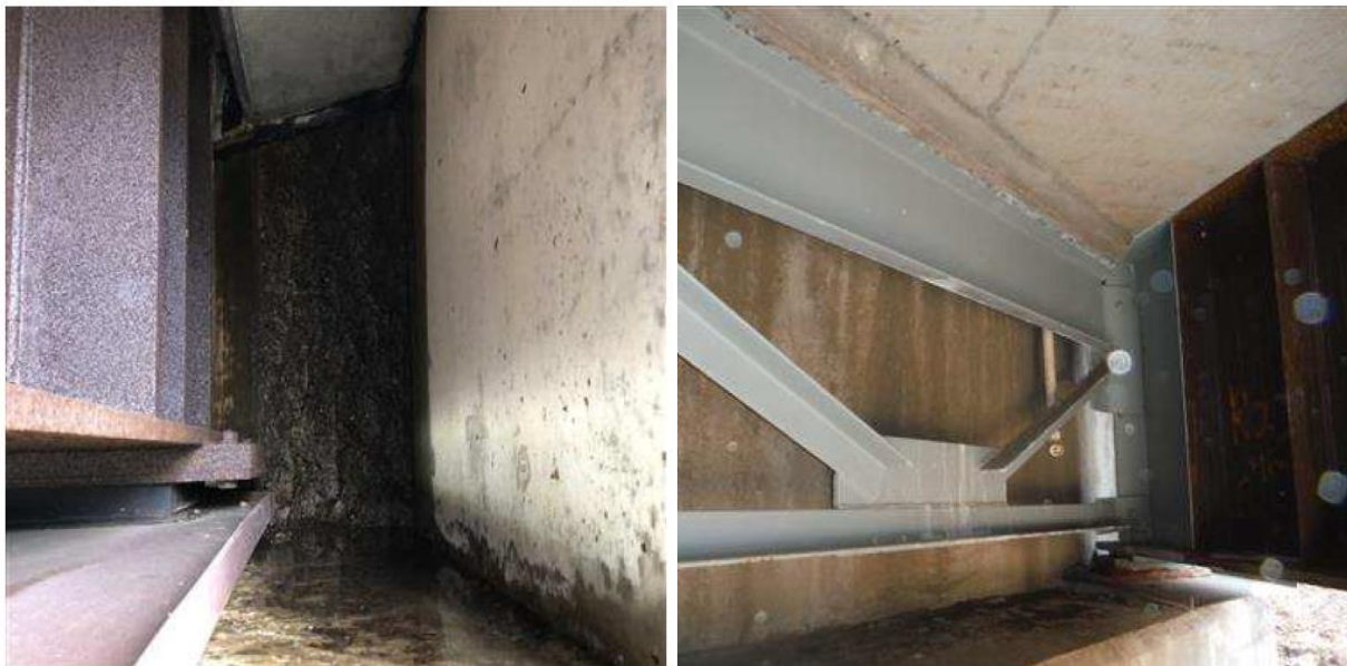
Figure 9. Examples of the Two Types of Beam End Leaking
