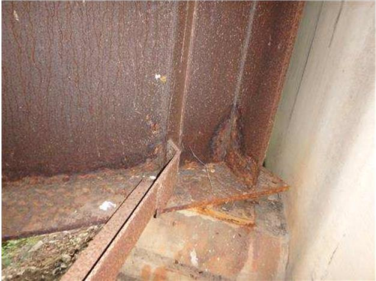
Figure 15. Example Section Loss at the Beam End
